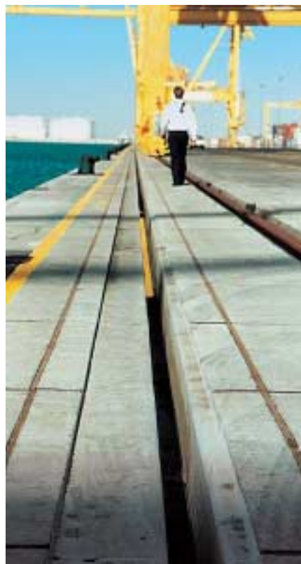
Jebel Ali Port - Dubai. The pre-existing slot used for the Panzerbelt installation.
