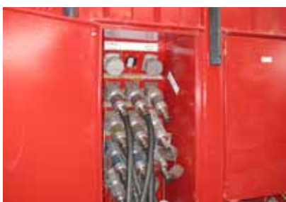
Power supply container on oil rig
