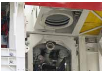
Power supply cables for top drive on oil rig
