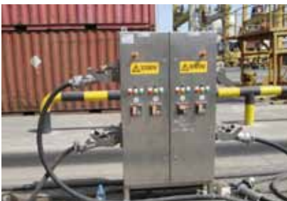
Ground mounted Power unit
